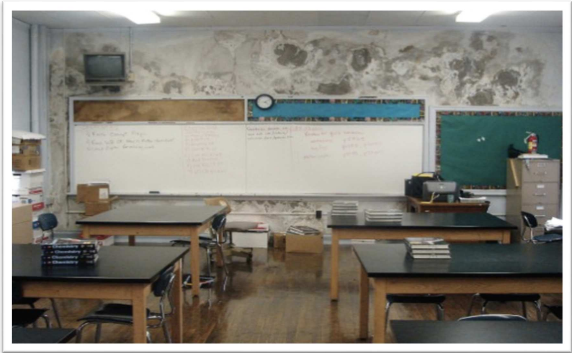
Photo: Water damage in a neighborhood school classroom.
