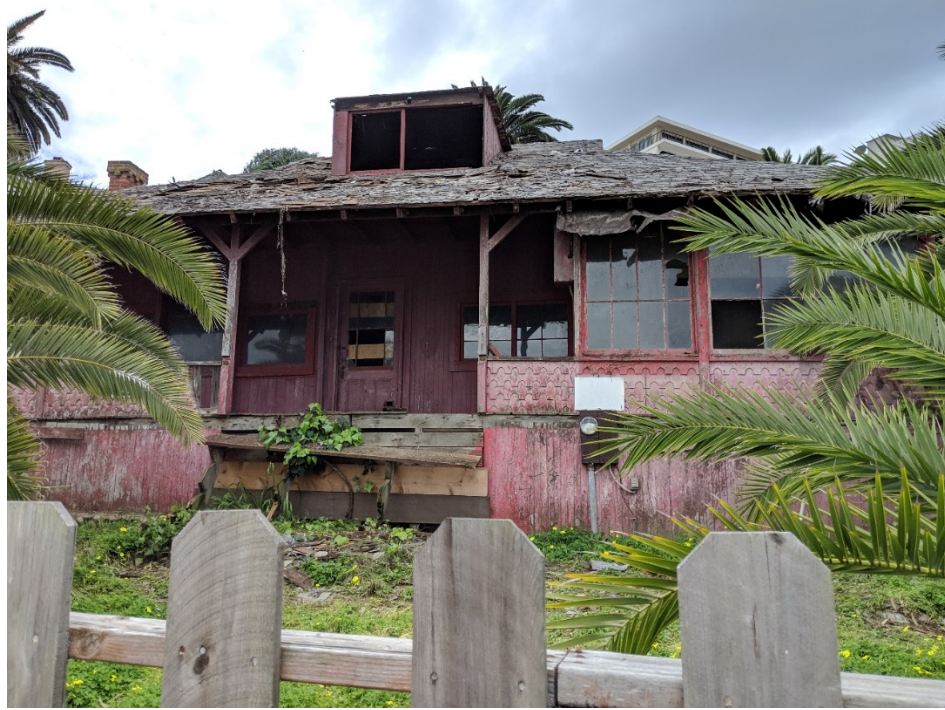
Figure 2.1 Red Rest Cottage, along with its neighbor Red Roost Cottage, is a rare example of a late-19 th century bungalow in La Jolla, California, but is currently suffering from demolition by neglect. (Photo by Jeff Scott, 2019)
