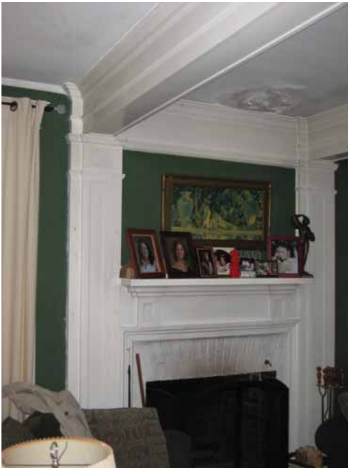
Figure 4.6: The existing living room fire places with beams extending from the fireplace surround. (Author's photograph)
