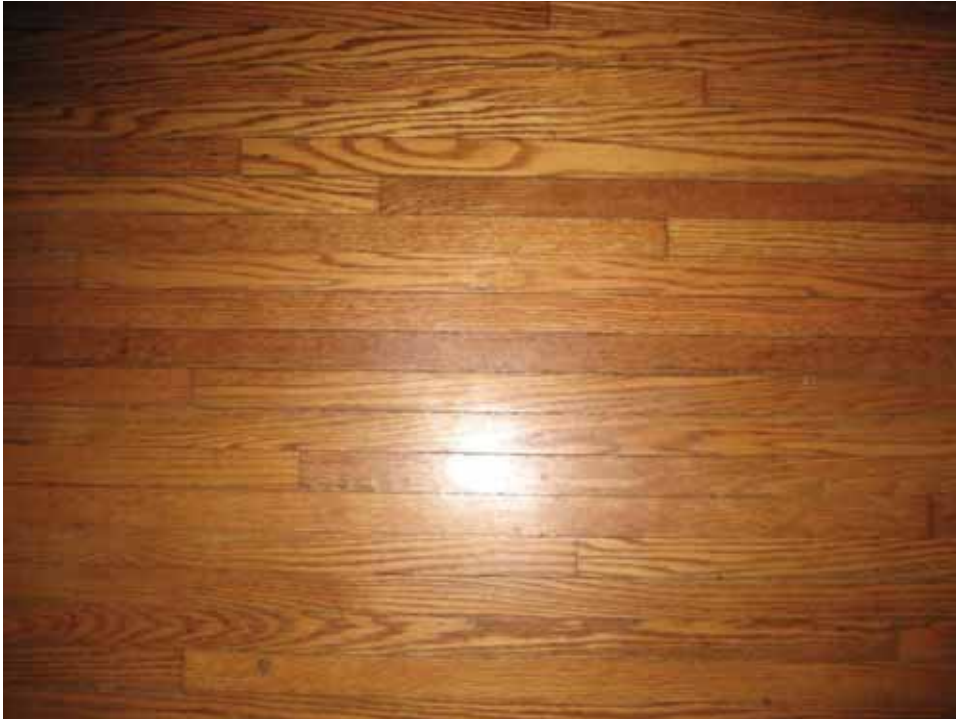
Figure 4.14: The existing hardwood floors of the living and dining rooms; one and a half to two inches wide. (Author's photograph)
