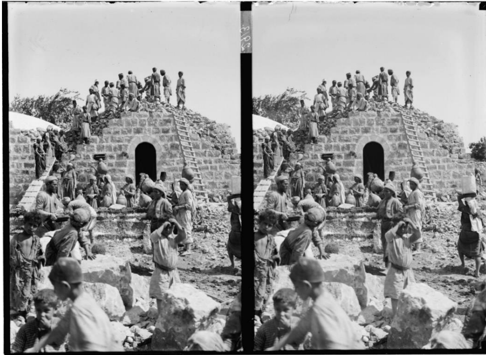
Fig. 5.5 “Building Stone House in Village in Hill Country.” Stenograph of communal building practices in early 20 th century Palestine. Photographer Unknown, Matson Collection, Library of Congress.
