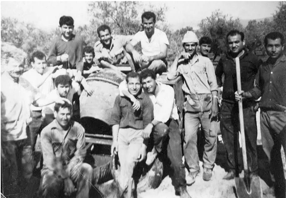
Fig. 5.6 Ibrahim Shamsoum and friends gathering around a cement mixer during the construction of Ibrahim’s house, 1965. Photo courtesy of the Shamsoum family.
