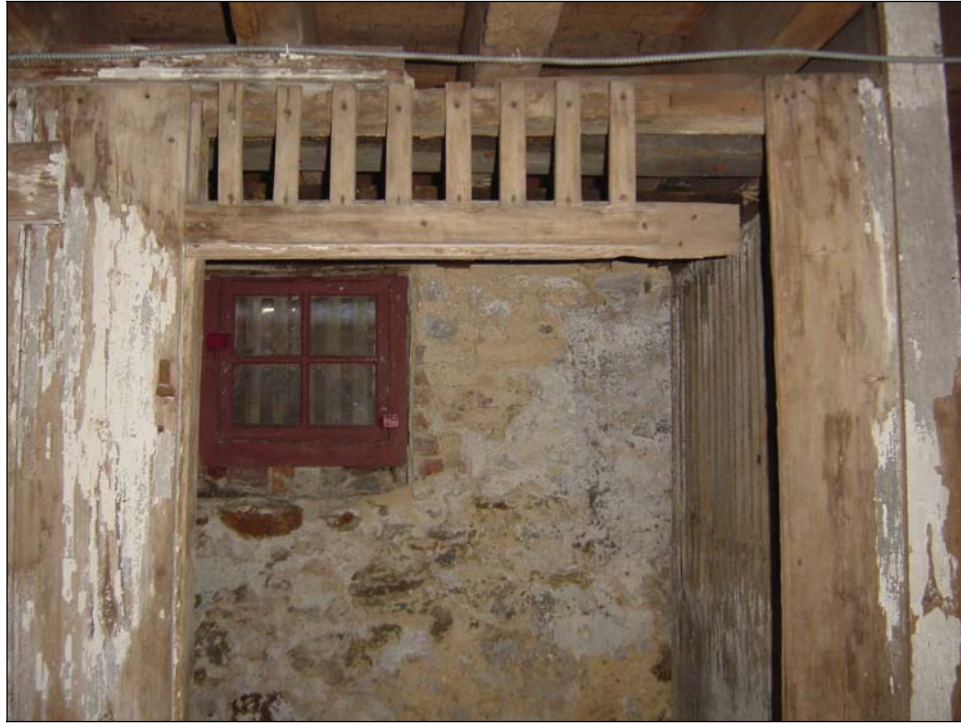
Figure 5: Ventilated window in closet in Northeast room (Higgins, 2006).
