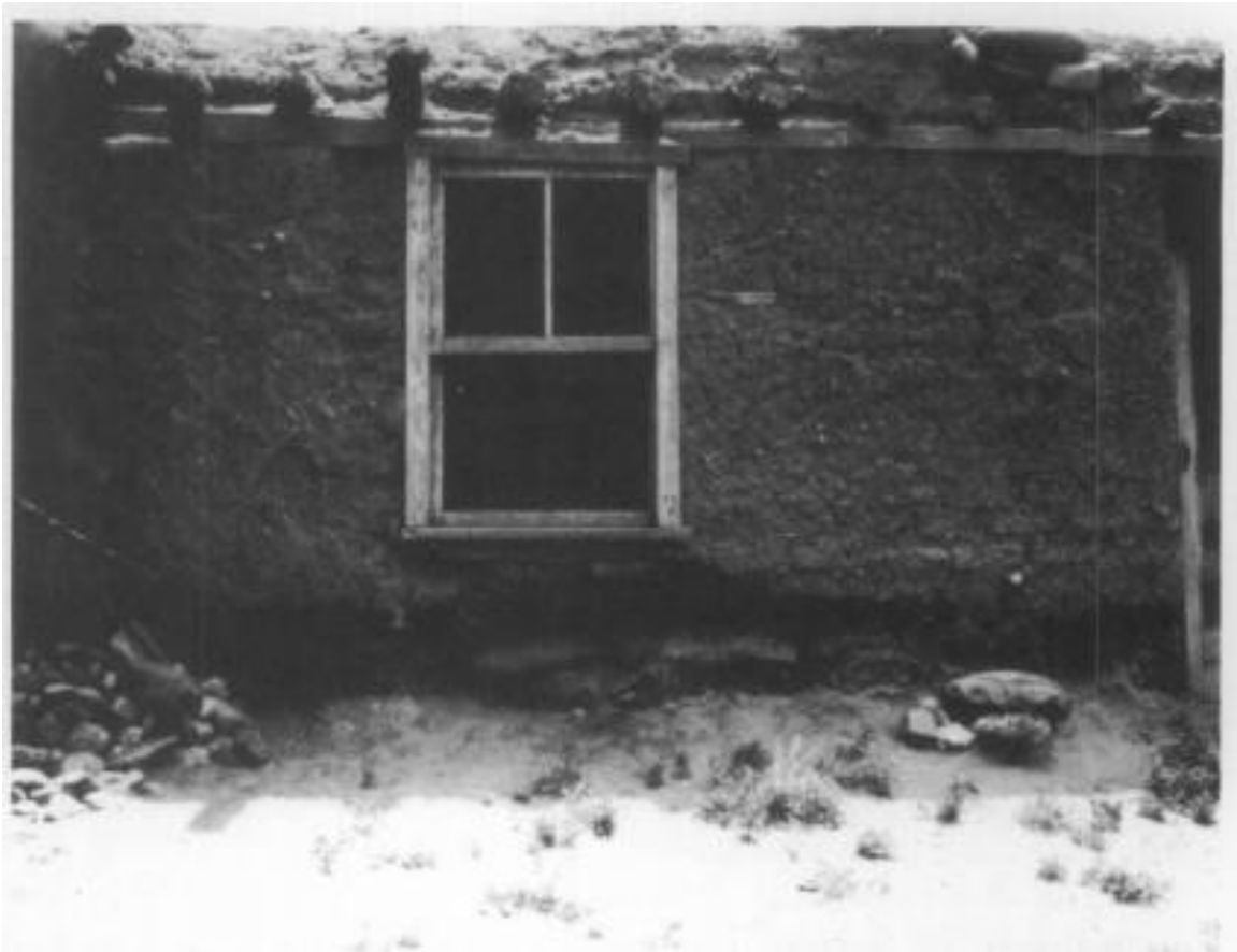
Figure 3.2: base erosion. image from National Park Service
