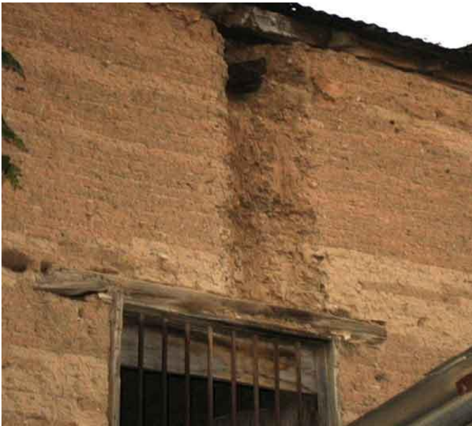
Figure 3.3: deterioration at the top of adobe walls. Image available online
