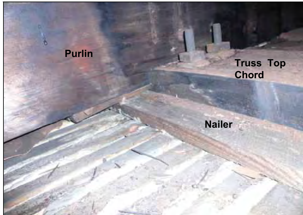
Figure 13: Roof probe 2, showing intersection of the purlins, nailers and truss. Photo by M. Goeke, 2007.
