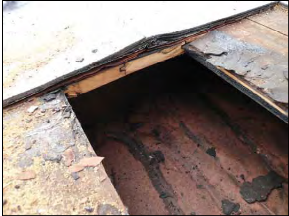
Figure 10: Probe 2, above area of water staining and displacement. Note the layers of roofing material and the water damage to the roof paper. Photo by M. Goeke, 2007.
