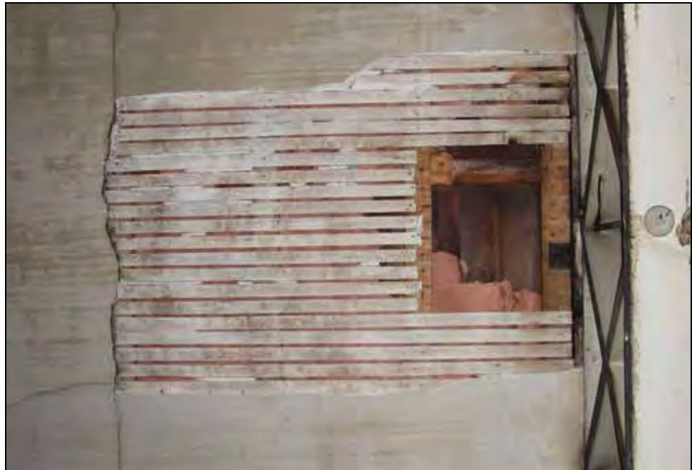
Figure 14: Area of loss in Bay 2. A nailer abuts the top chord of the truss. They then are set 16 inches apart. Lath spacing, some too close together, is also visible. Photo by A. Finke, 2007.
