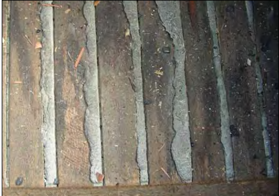
Figure 15: Probe 2. Gaps between lath and plaster may indicate drying and shrinking of the wood. Photo by A. Finke, 2007.
