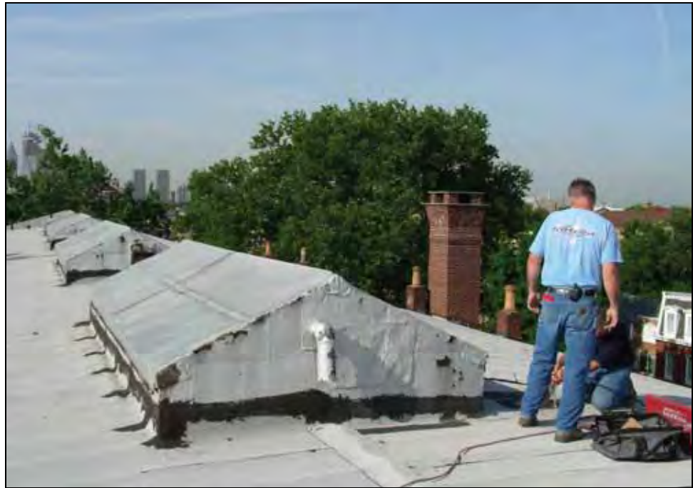
Figure 16: Skylights from the roof. Note the patching around the edge of the skylights. Photo by A. Finke, 2007.
