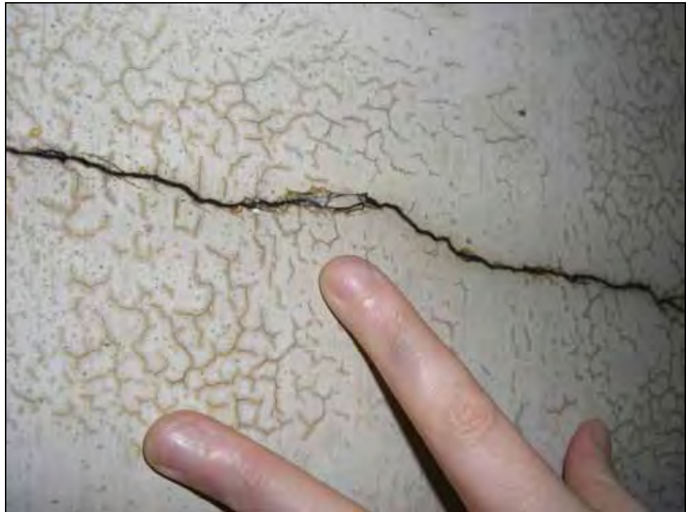
Figure 9: Large crack. Photo by M. Goeke, 2008.
