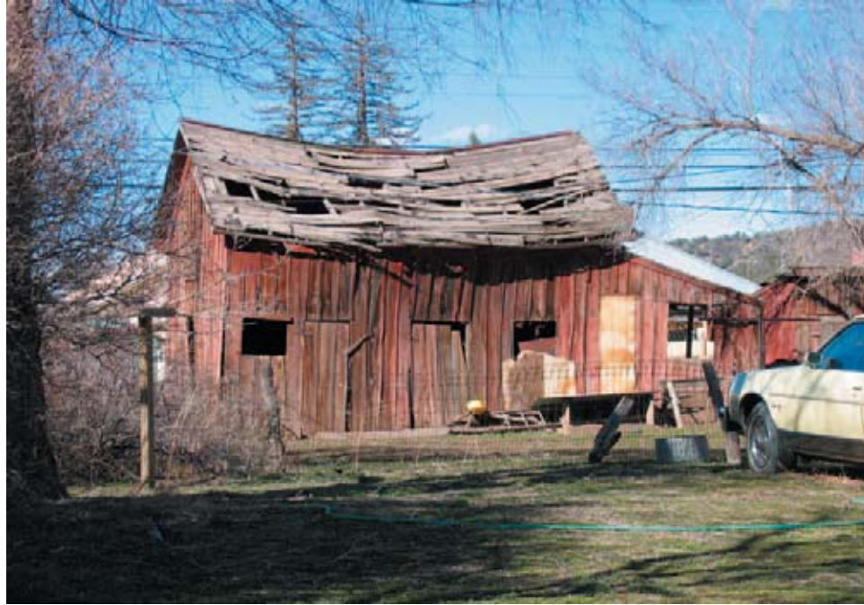
Figure 43-Small Wooden Structure in Disrepair, Mancos, 2005
