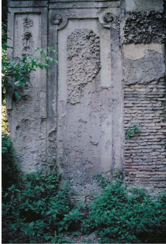
Figure 7.5: Example of damage to spugne textured surface caused by roots; also visible on right is missing plaster and exposed brick. (Sardegna, 2002)
