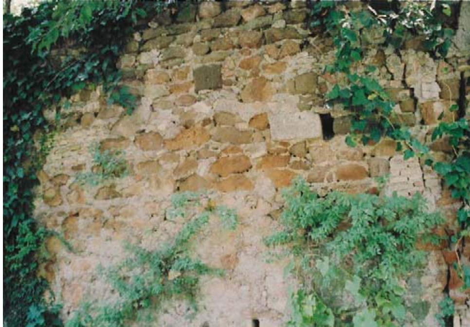
Figure 2.2: Typical tuff stone ranging in color from buff to yellow in the old scalinata walls. (Sardegna, 2002)
