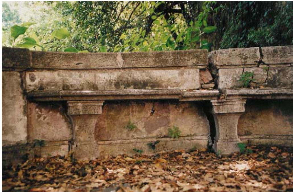
Figure 7.3: Displaced masonry on the scalinata near the plane trees. (Sardegna, 2002)
