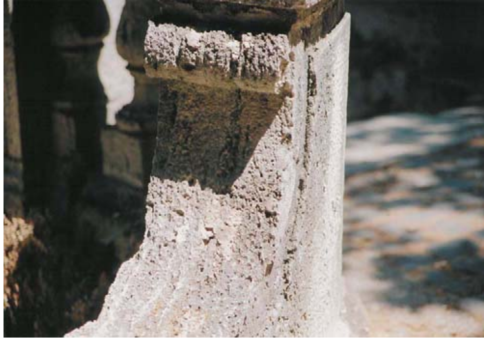
Figure 7.2: Pitted travertine surface on the scalinata baluster. (Sardegna, 2002)
