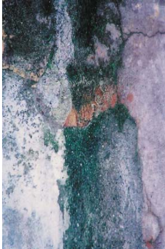
Figure 5.13: Exposed site of sample SC-012. The grey field below the exposed orange finish plaster appears to be a more recent repair.
