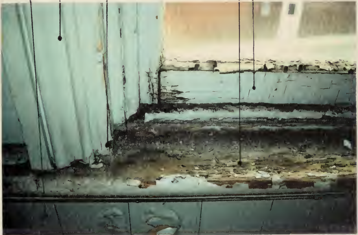
Illustration 16 View of the main corridor in the Female Grammar School showing the existing condition of interior materials
