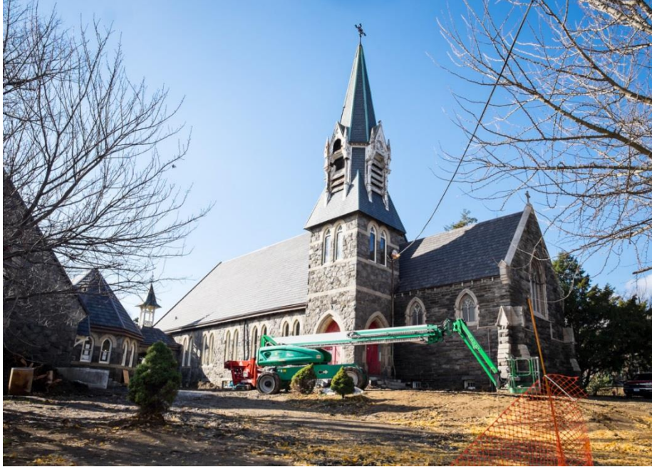
Figure 14: St. Peter's Episcopal Church, 2014. This image shows the physical condition of the main church building on the St. Peter's Episcopal Church property, after some stabilization and preventative maintenance has occurred. The exterior is similar to the how it would have appeared in 2011, when Weinstein first acquired the property. The image comes from the Waldorf School of Philadelphia's blog, "Loving Learning".
