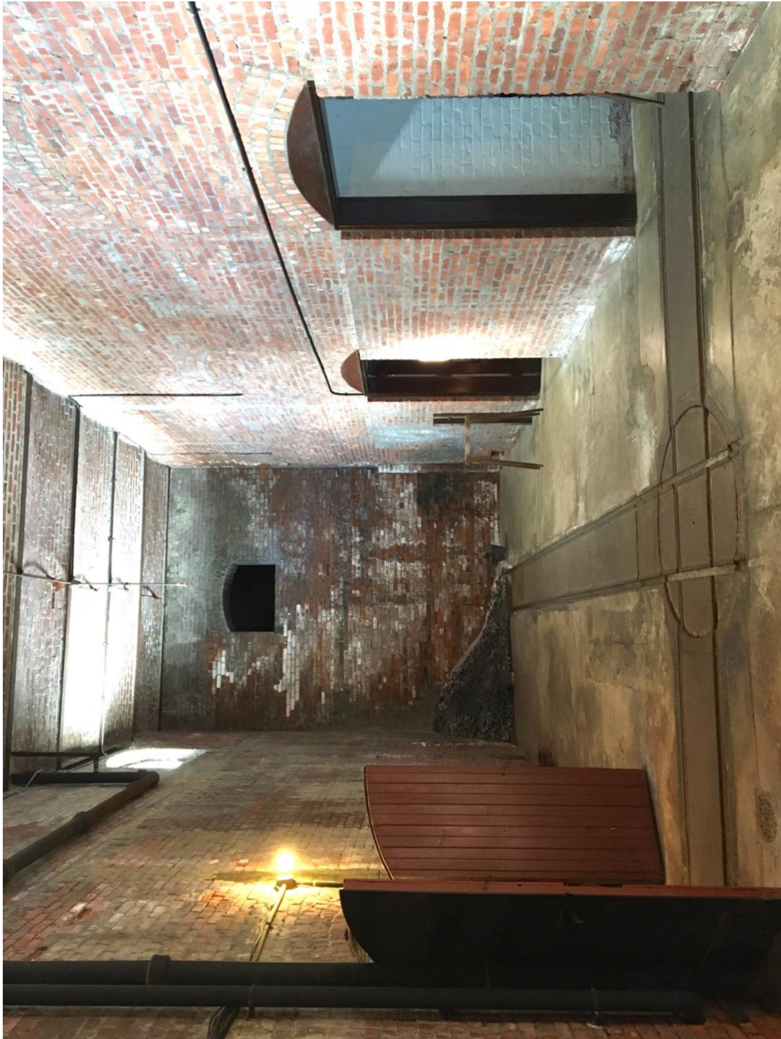
Figure 15: The coal room in The Elms sub-basement. The entrance to the tunnel is on the left, the coal storage area is directly ahead, and the doorway to the boilers is on the right. Photo by author.
