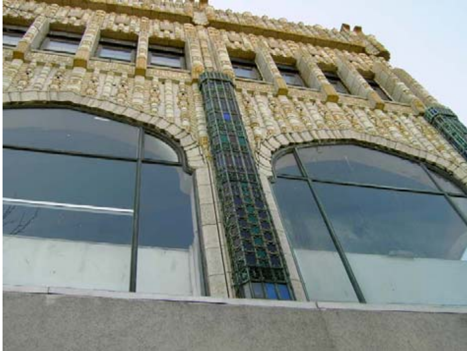
Figure 5. Second and third stories, as viewed from 69 th Street (photograph by author)
