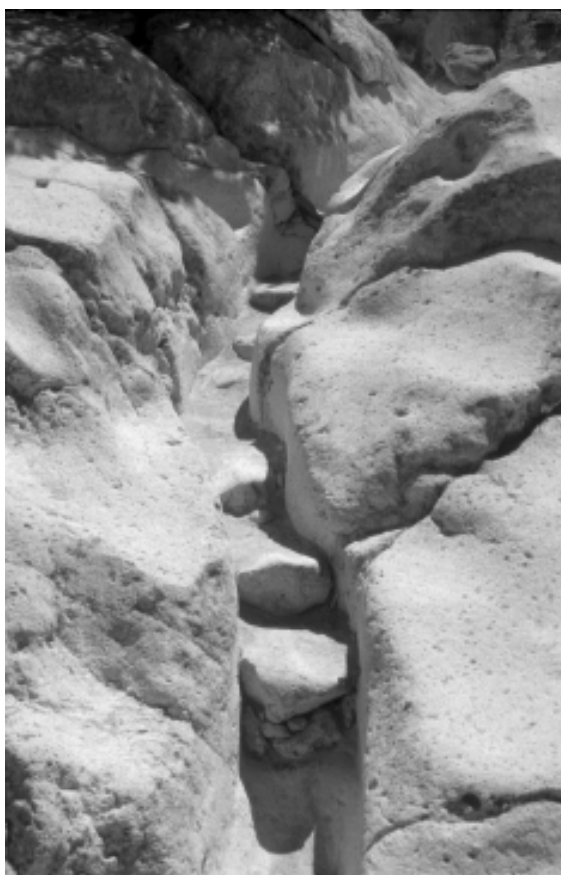
Figure 14. Deeply eroded trail, after stabilization with compacted gravel and added rock retaining steps.
