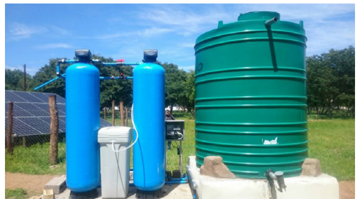
Figure 5: Water filtration system for Igusi Clinic and nearby school in 2019, Source: J.B. Dondolo, Inc. (2021)
