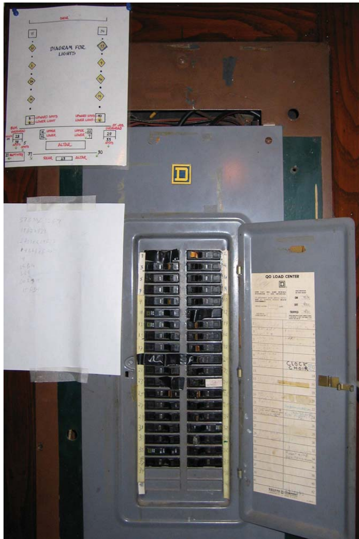
Figure 5: A circuit breaker panel in St. Agatha-St. James Roman Catholic Church in Philadelphia. Most of the luminaires in the church are controlled from this panel, but many are controlled from other isolated switches, including one located just above the floor in one of the side altar areas. Note the diagram to help make sense of which switches control which luminaires, and the electrician's tape covering some of the switches as a way to keep them either always on or always off.
